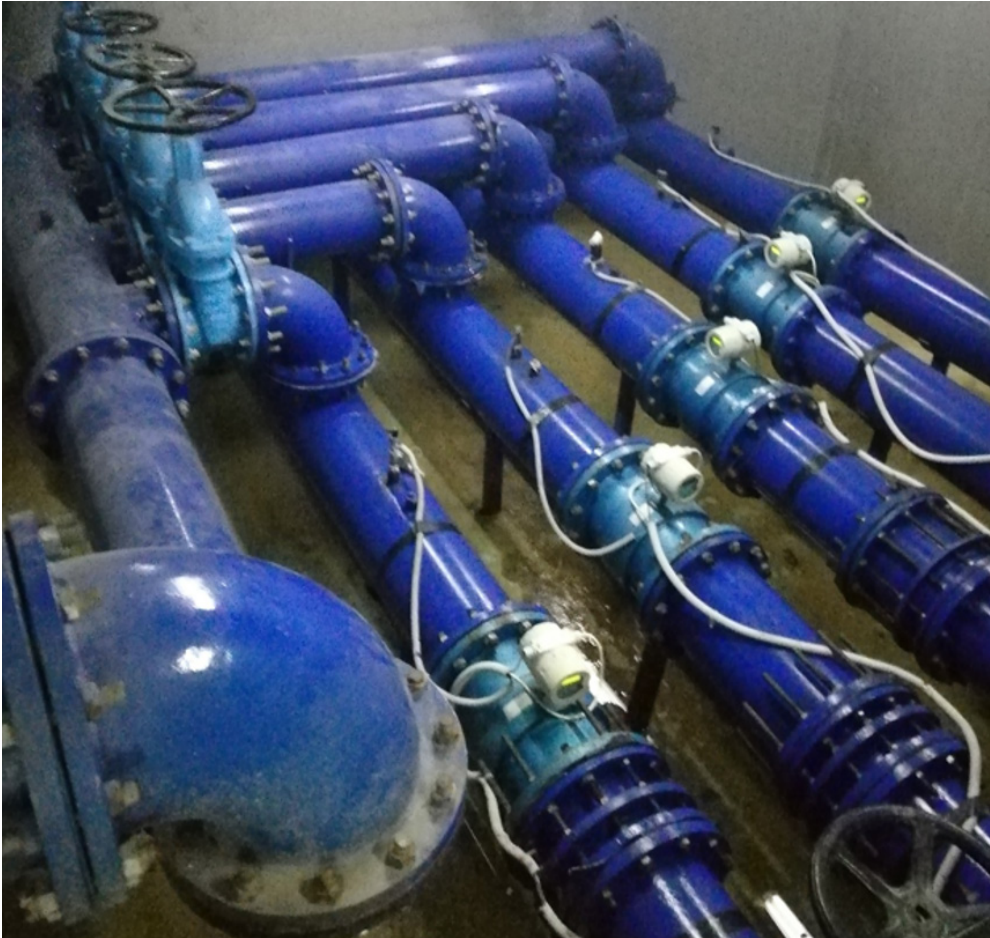
Figure 41. Madiq pumping station
