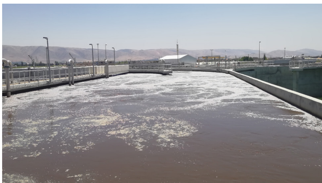
Figure 79. Zahle wastewater treatment plant
