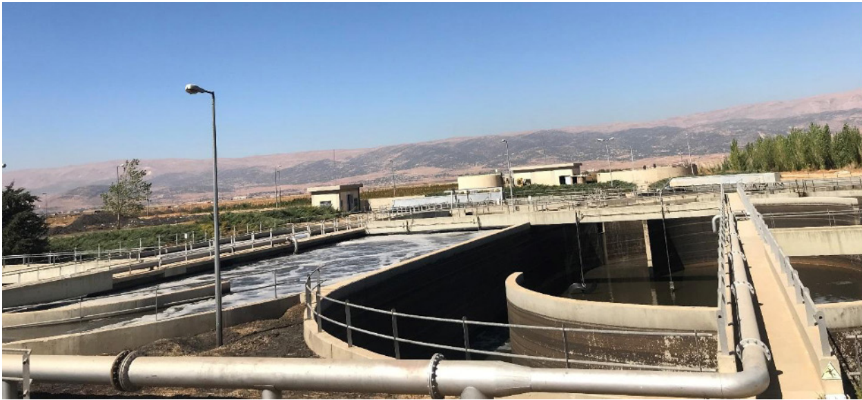
Figure 80. laat wastewater treatment plant
