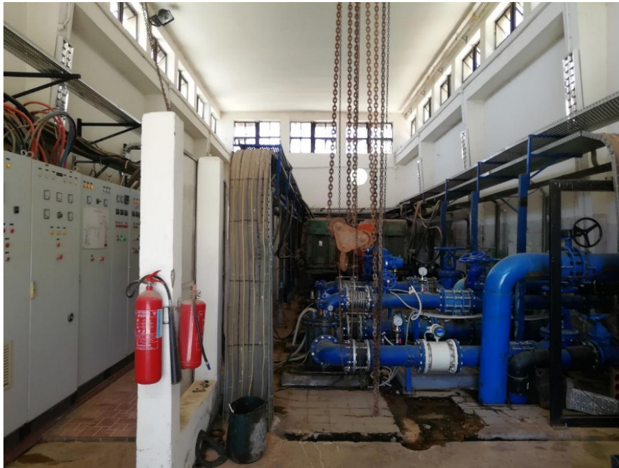
Figure 36. Loussi water pumping station
