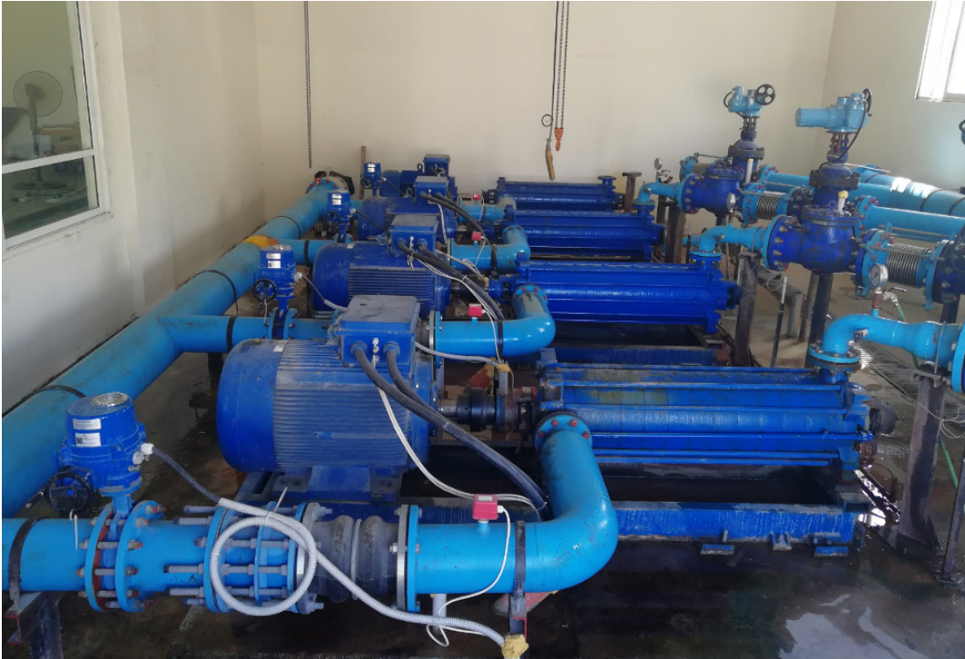
Figure 61. Chekka water pumping station
