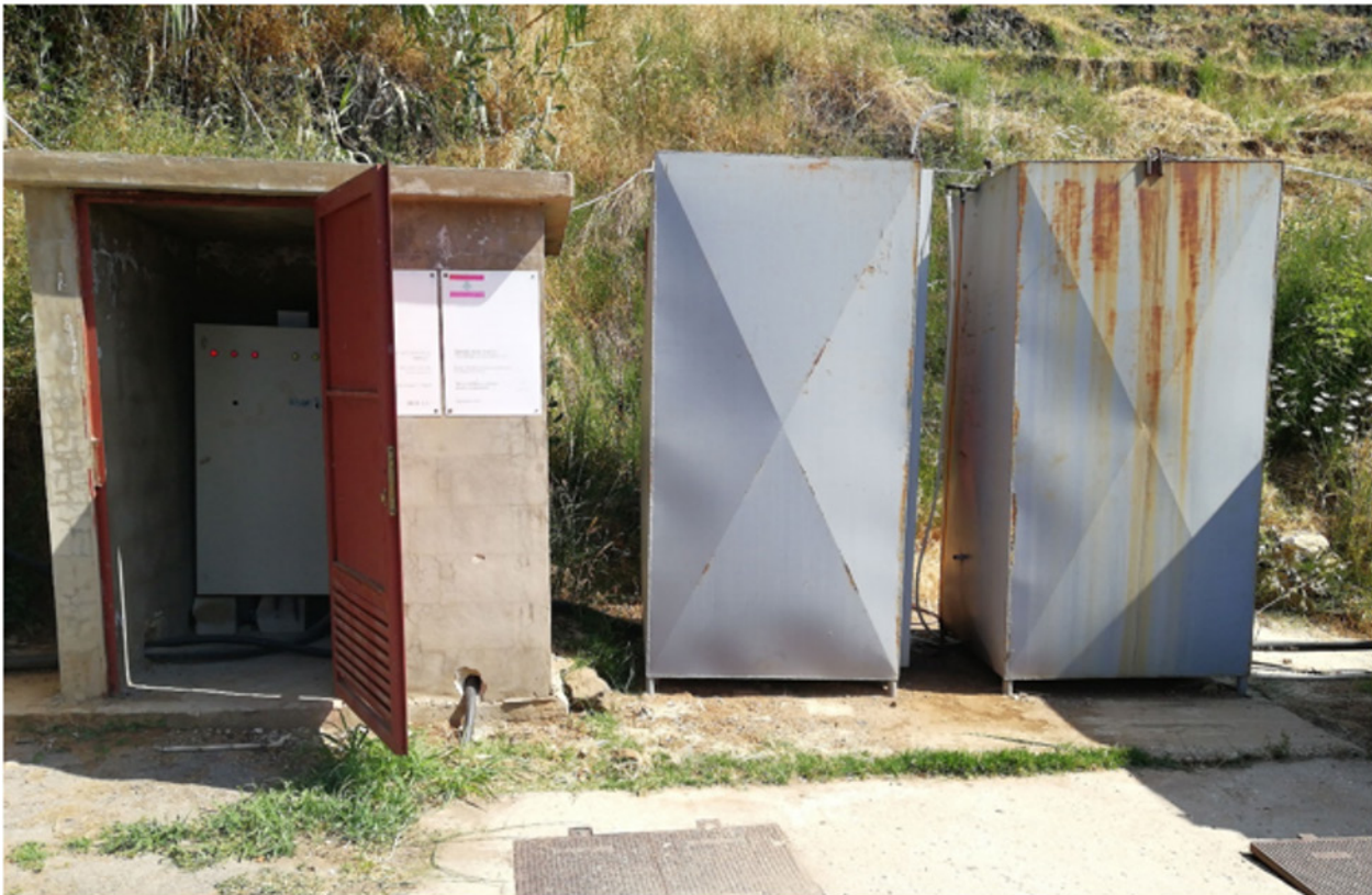
Figure 39. Qartaba pumping station
