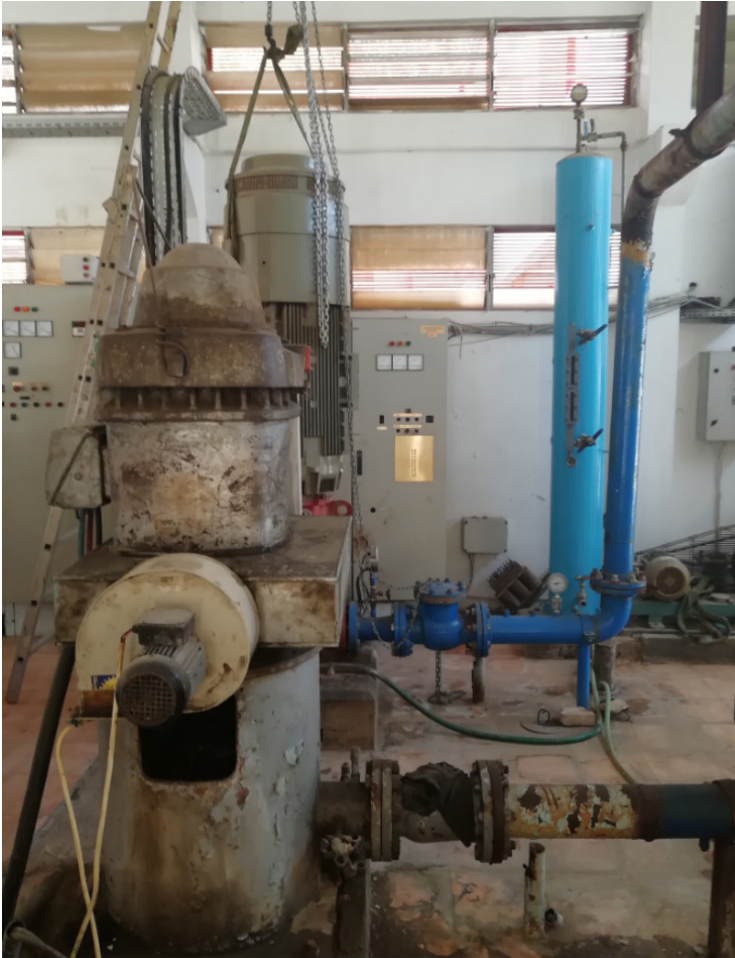
Figure 63. Kfarhelda water treatment plant
