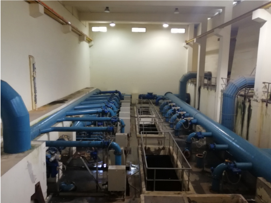
Figure 58. Al Manar Water pumping station
