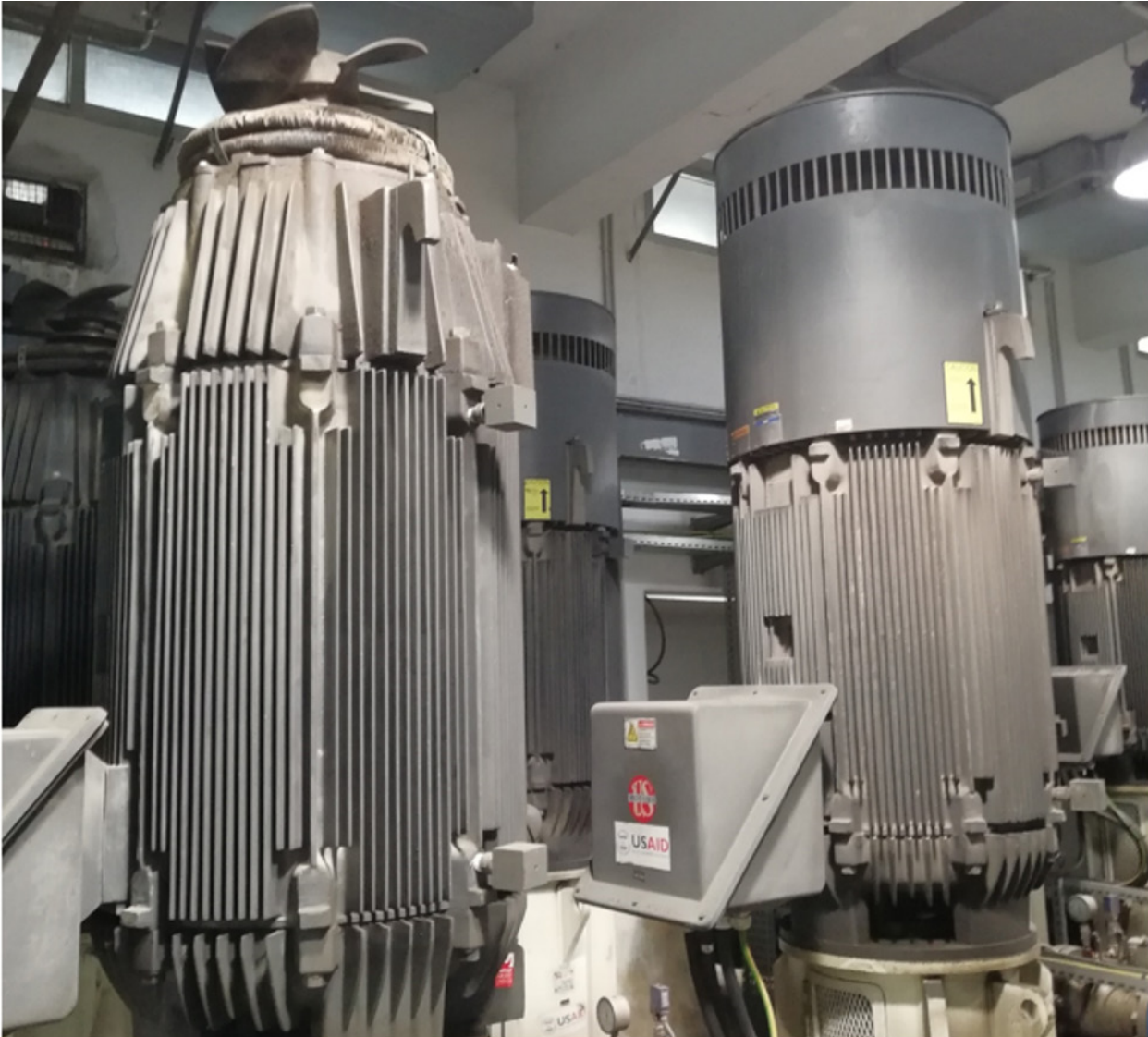
Figure 45. Jeita pumping station
