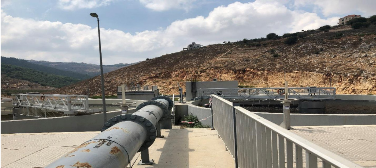
Figure 101. Tebnin wastewater treatment plant
