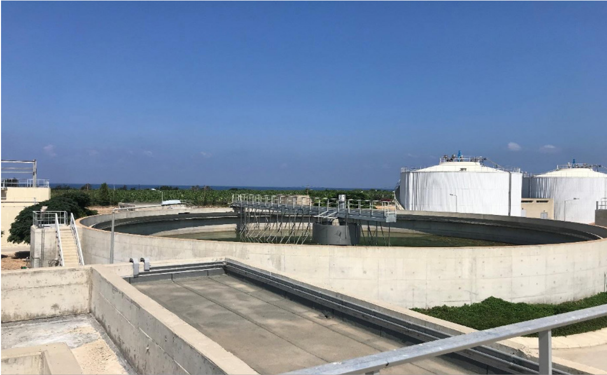
Figure 102. Sour wastewater treatment plant
