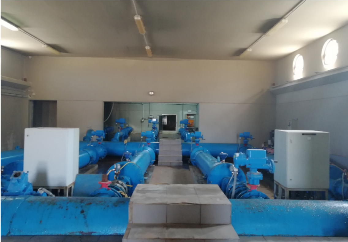
Figure 57. Abou Halka pumping station
