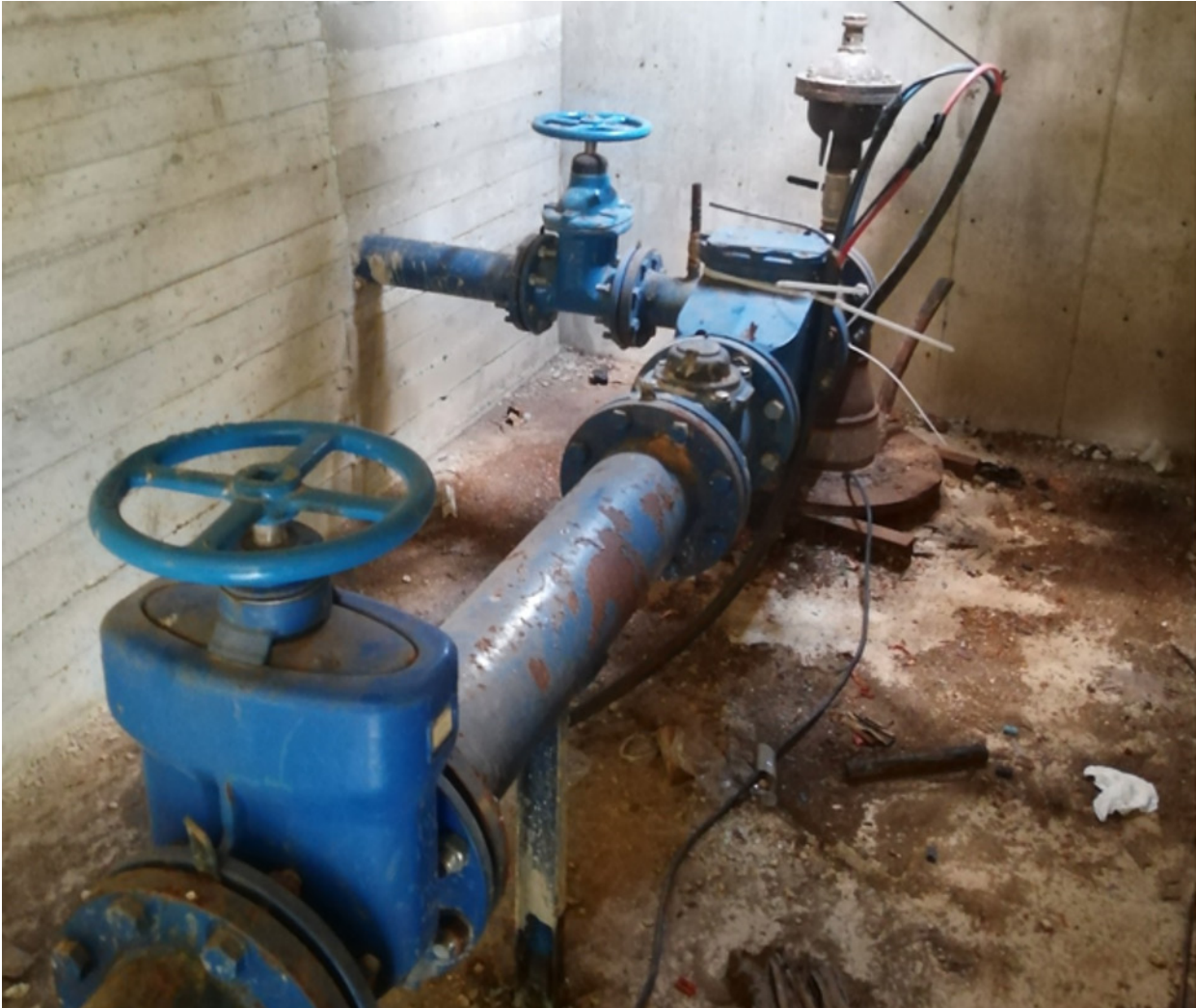
Figure 44. Qashqoush pumping station
