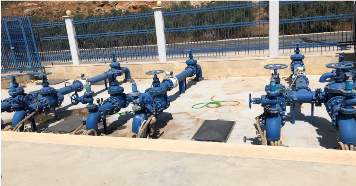
Figure 75. Marj El Khookh water pumping station
