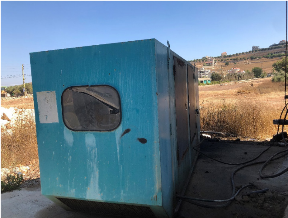
Figure 78. Maroun Al Ras station
