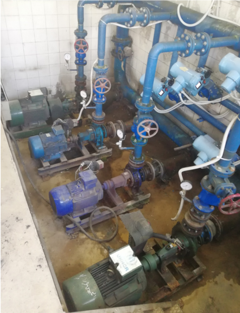
Figure 49. Jamhour pumping station
