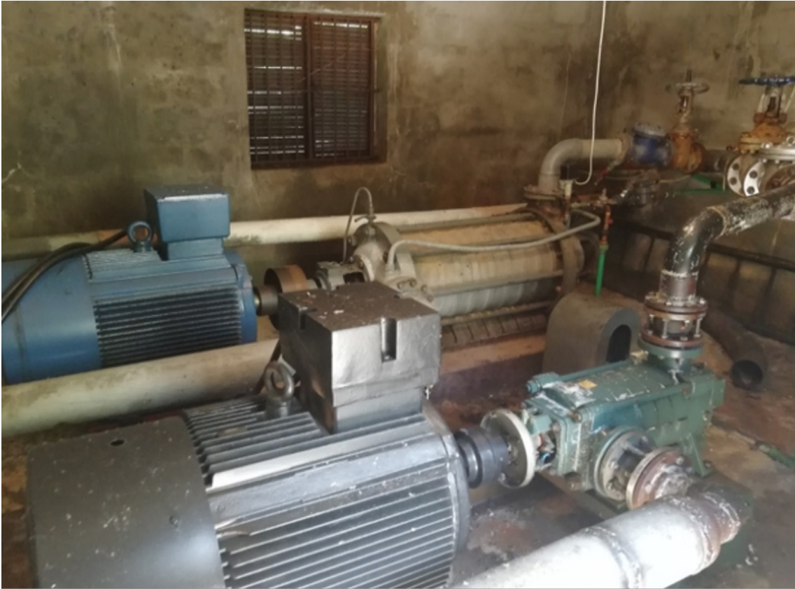
Figure 40. Akoura pumping station
