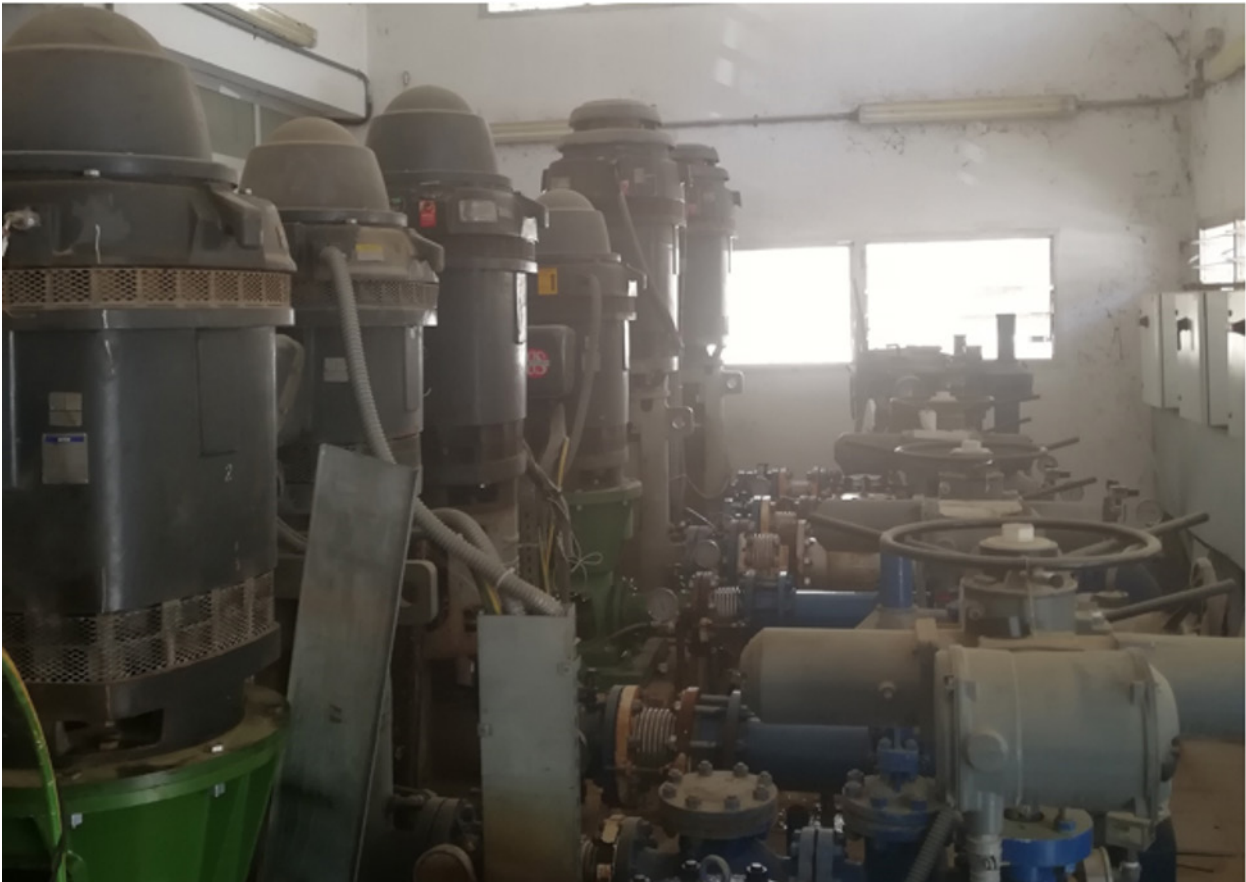
Figure 47. Nabaa El Safa pumping station
