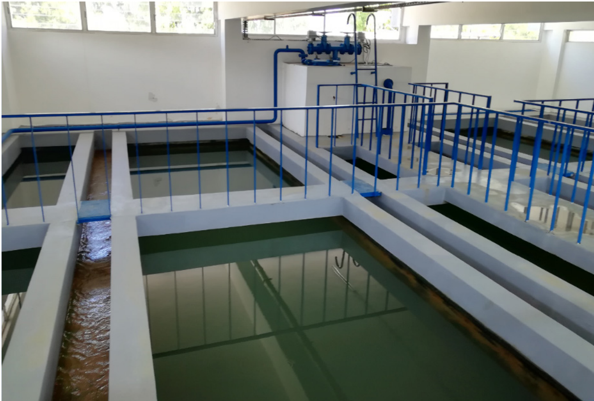
Figure 72. Ras El Ain Water Treatment Station
