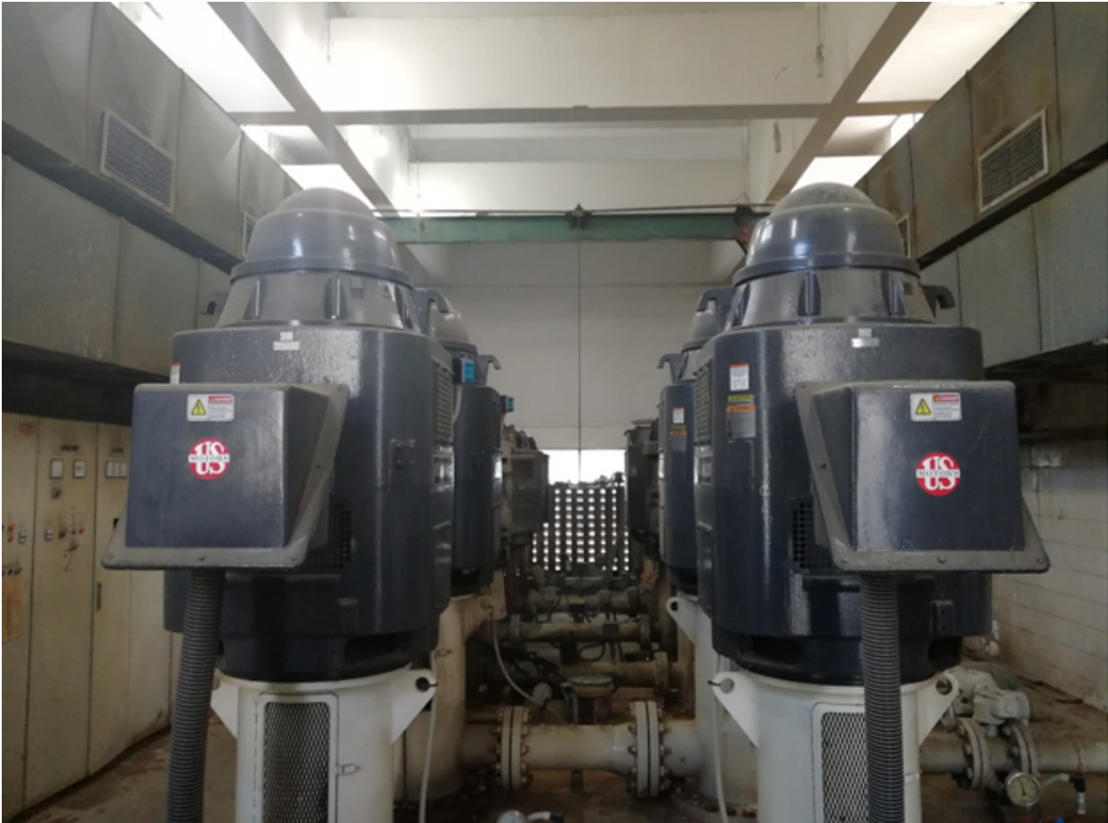
Figure 43. Qornet El Hamra pumping station
