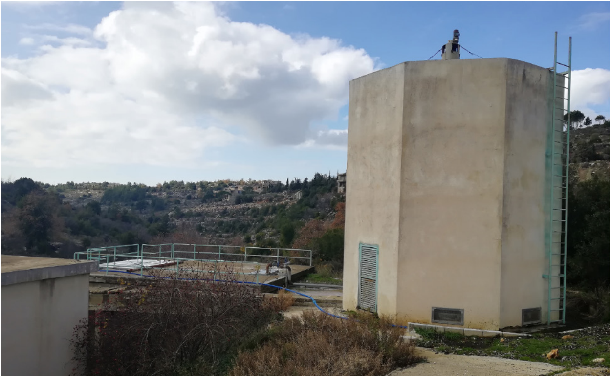
Figure 94. Maaser El Chouf wastewater treatment plant
