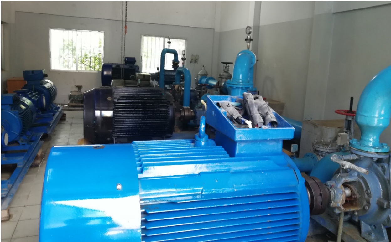
Figure 70. Fakhreddine Water Pumping Station
