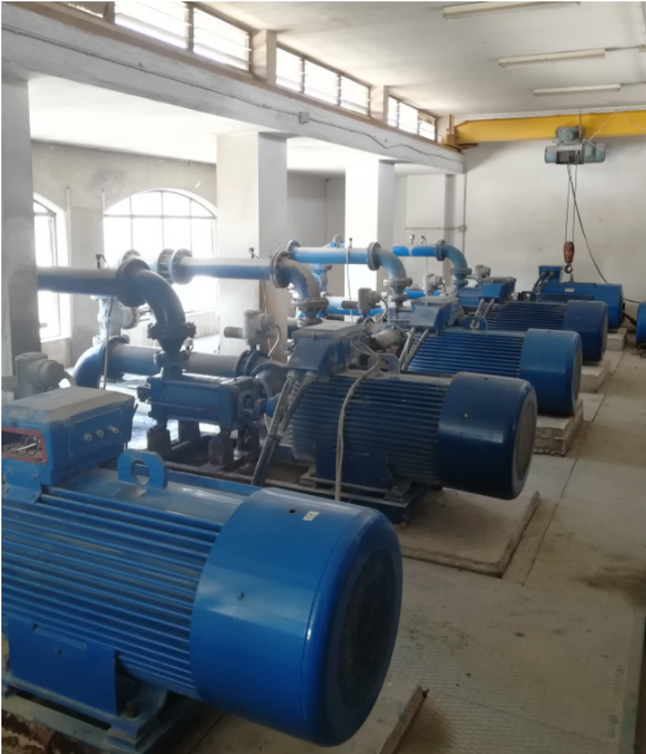
Figure 60. Jradeh Water pumping station
