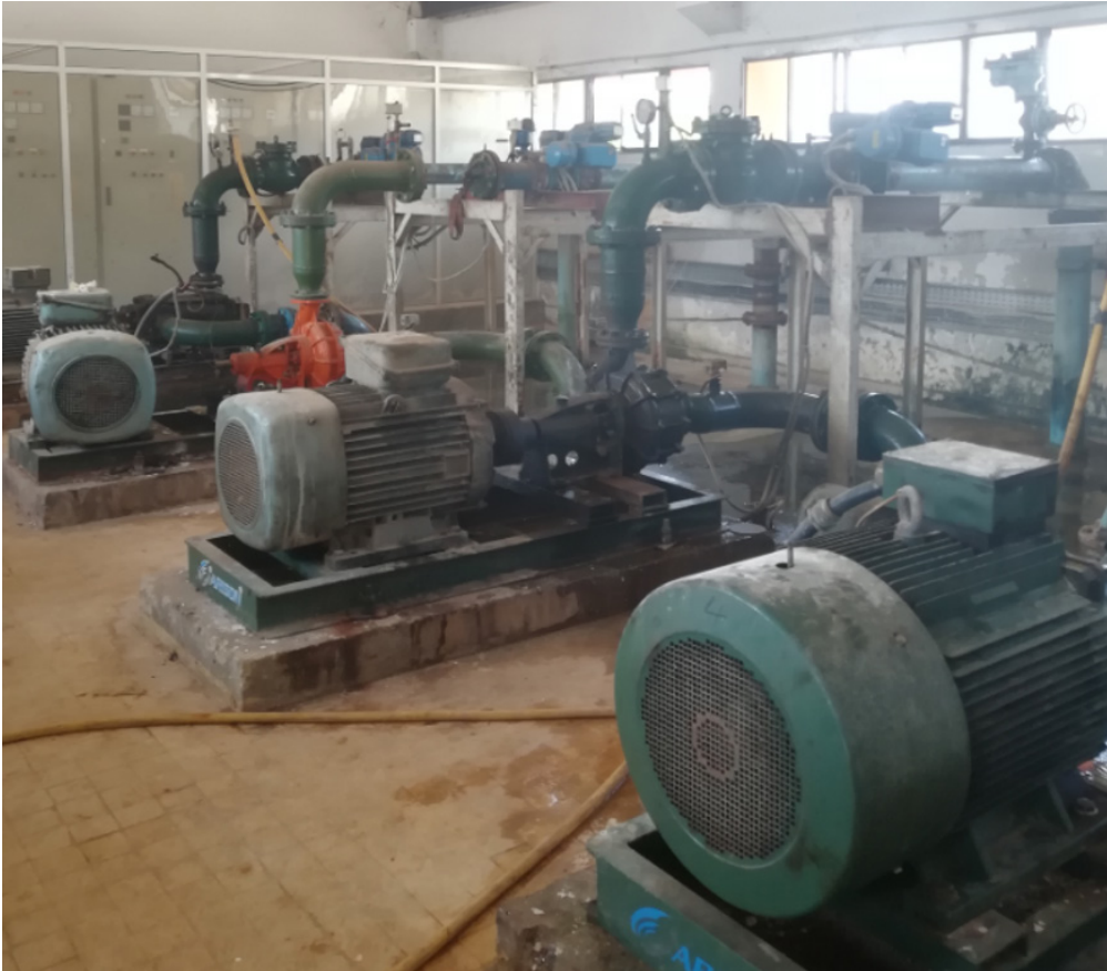
Figure 66. Al Kadi spring water pumping station
