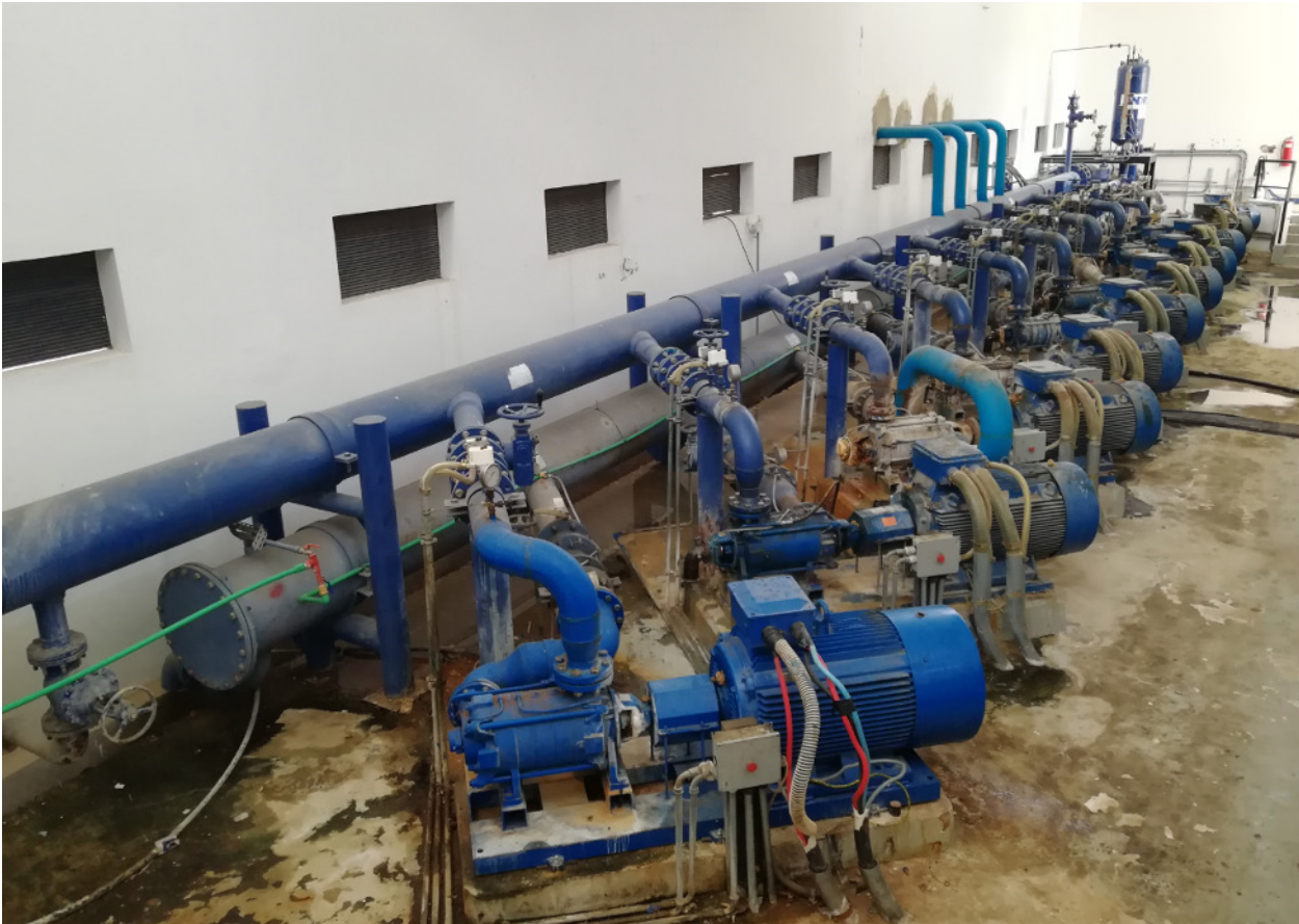
Figure 73. Wadi Jilo water pumping station
