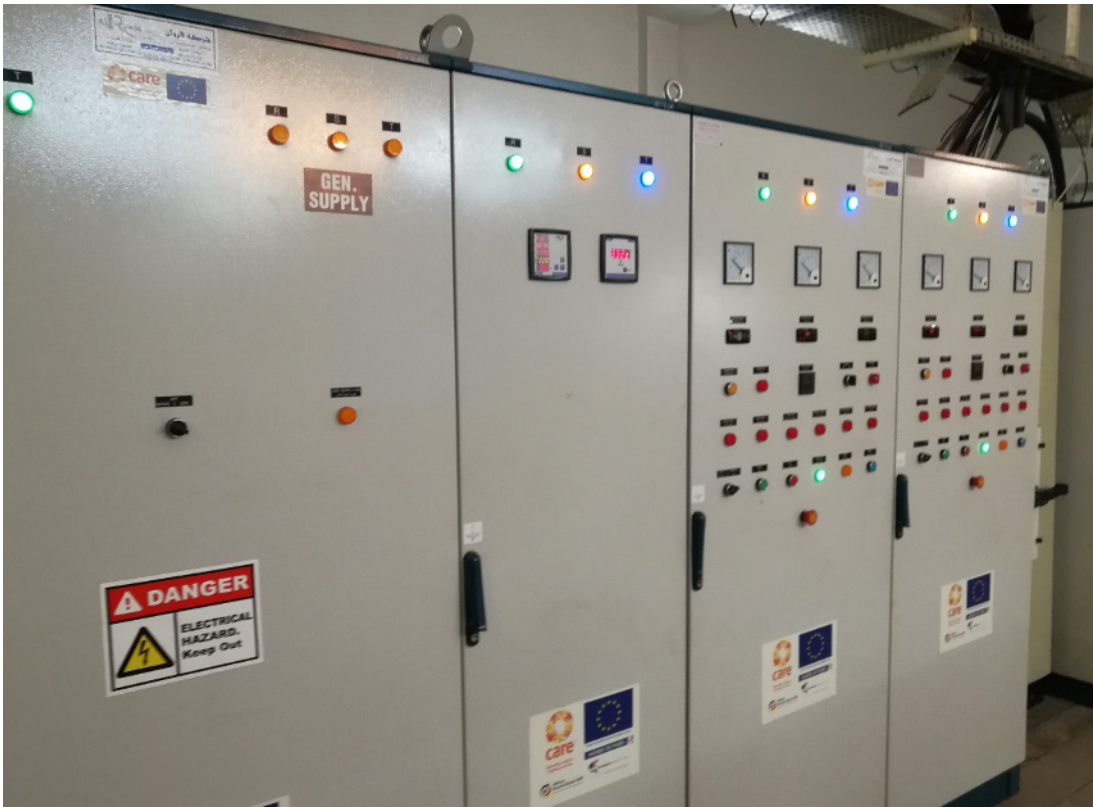
Figure 67. Arabi water pumping station
