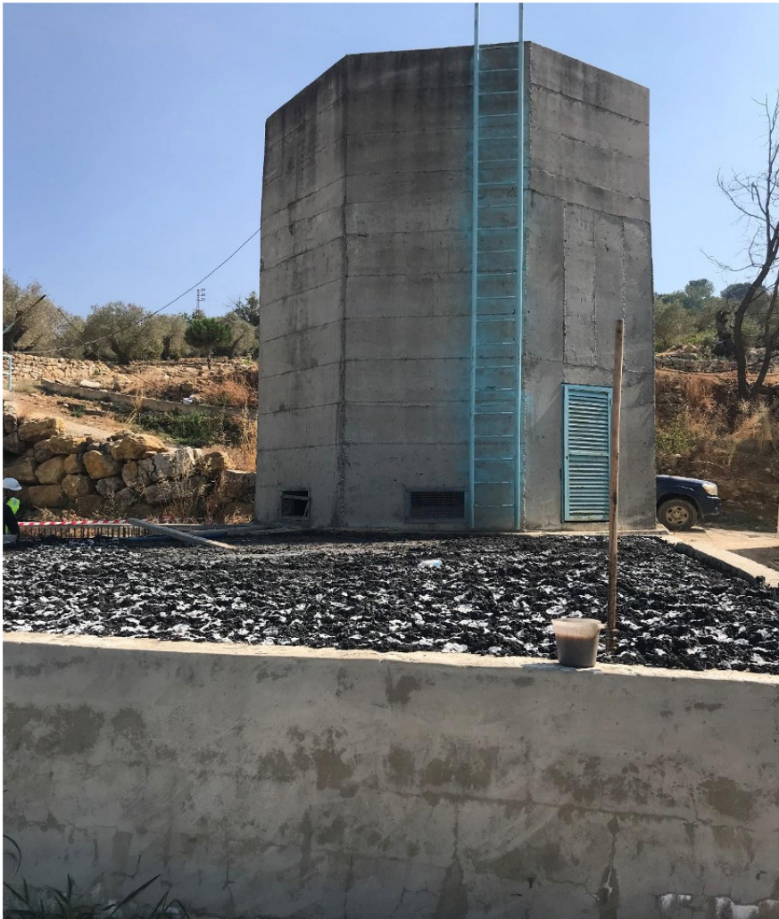
Figure 89. Mokhtara wastewater treatment plant
