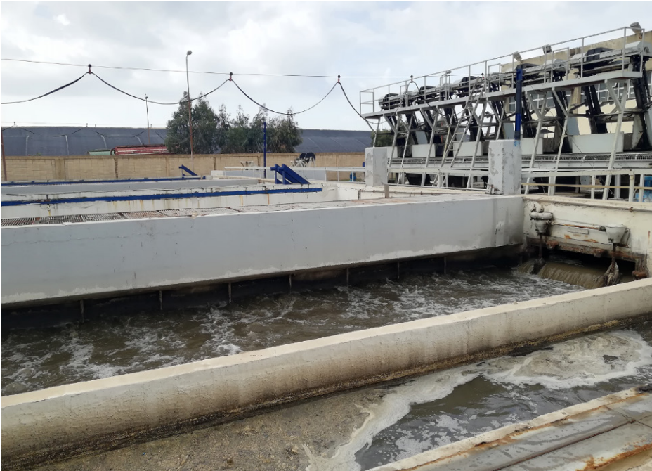
Figure 95. Ghadir wastewater treatment plant
