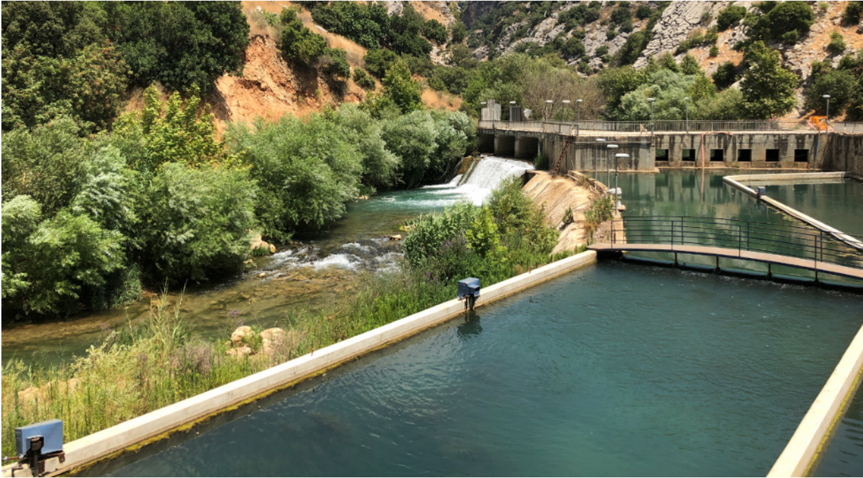
Figure 77. Taybeh River pumping station
