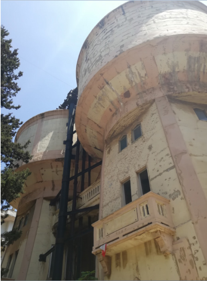
Figure 59. Abou Samra water pumping station
