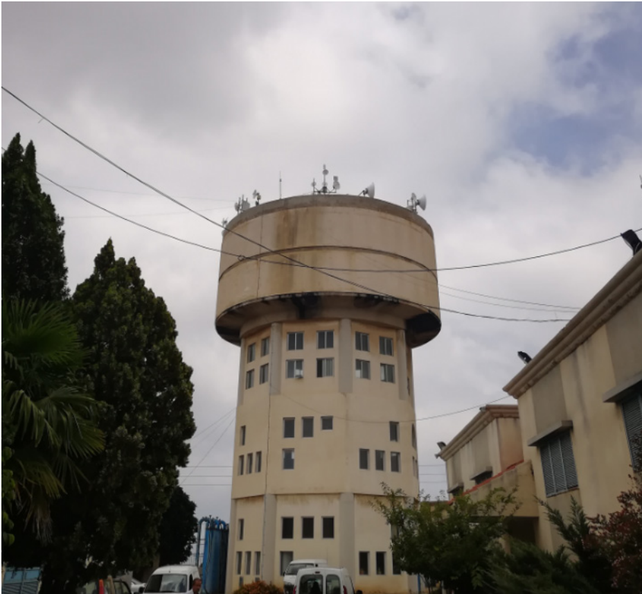
Figure 69. Teffahta water pumping station
