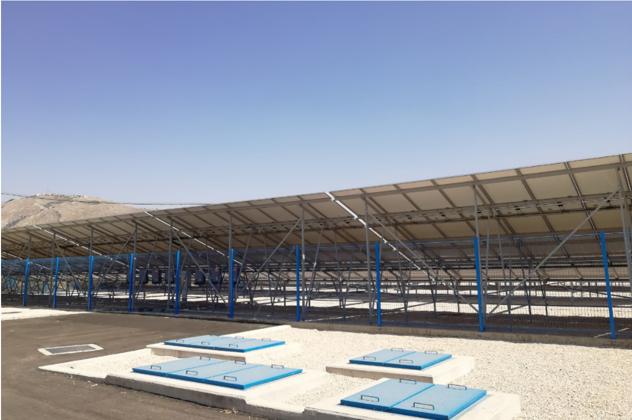
Figure 37. Ghazze solar pumping station
