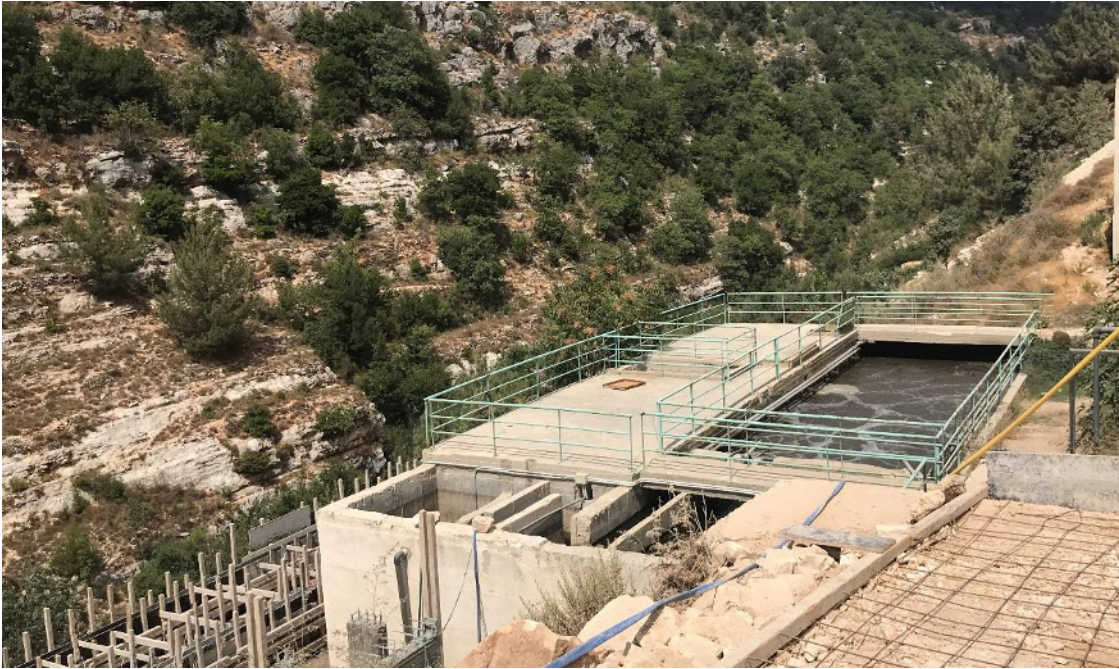
Figure 91. Mrosti wastewater treatment plant
