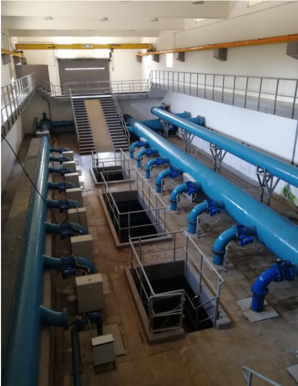
Figure 55. Ayrounieh water pumping station
