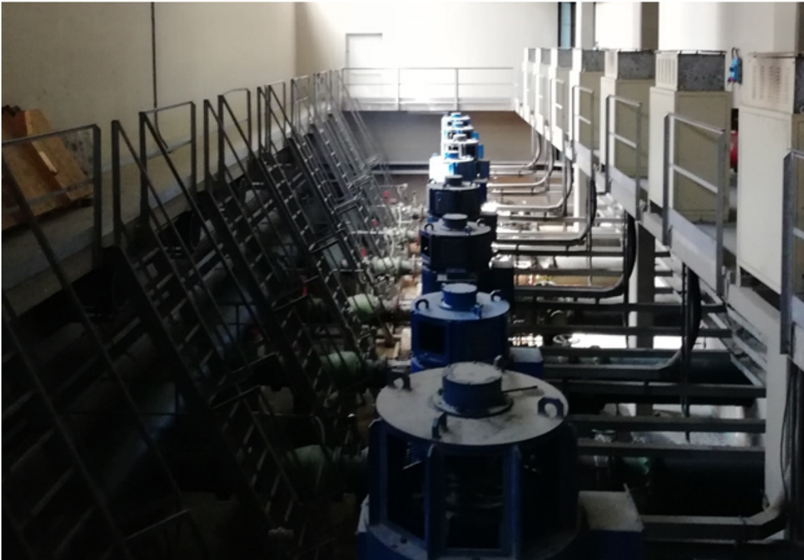
Figure 42. Ashrafieh pumping station
