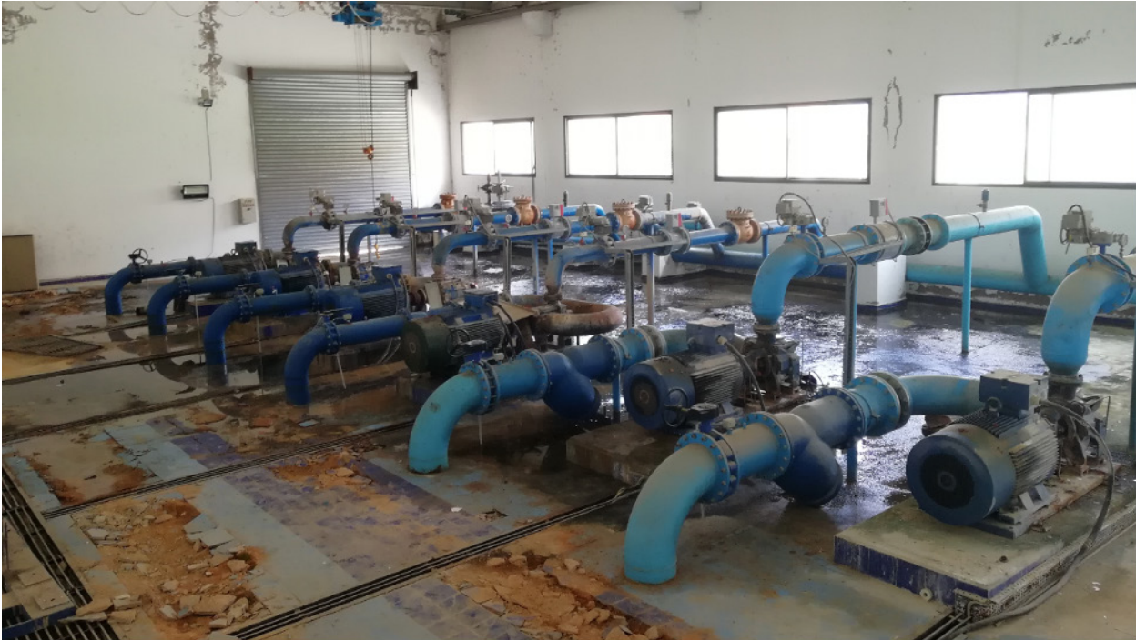
Figure 74. Yanouh water pumping station
