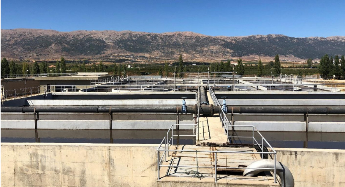
Figure 82. Jeb Jannine wastewater treatment plant
