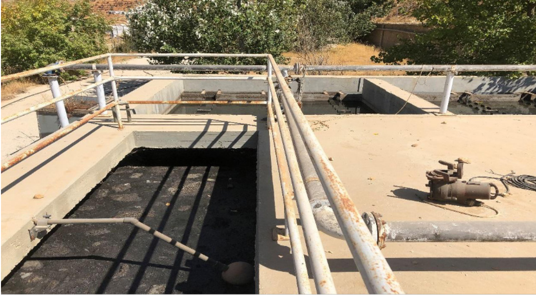
Figure 81. Yammouneh wastewater treatment plant
