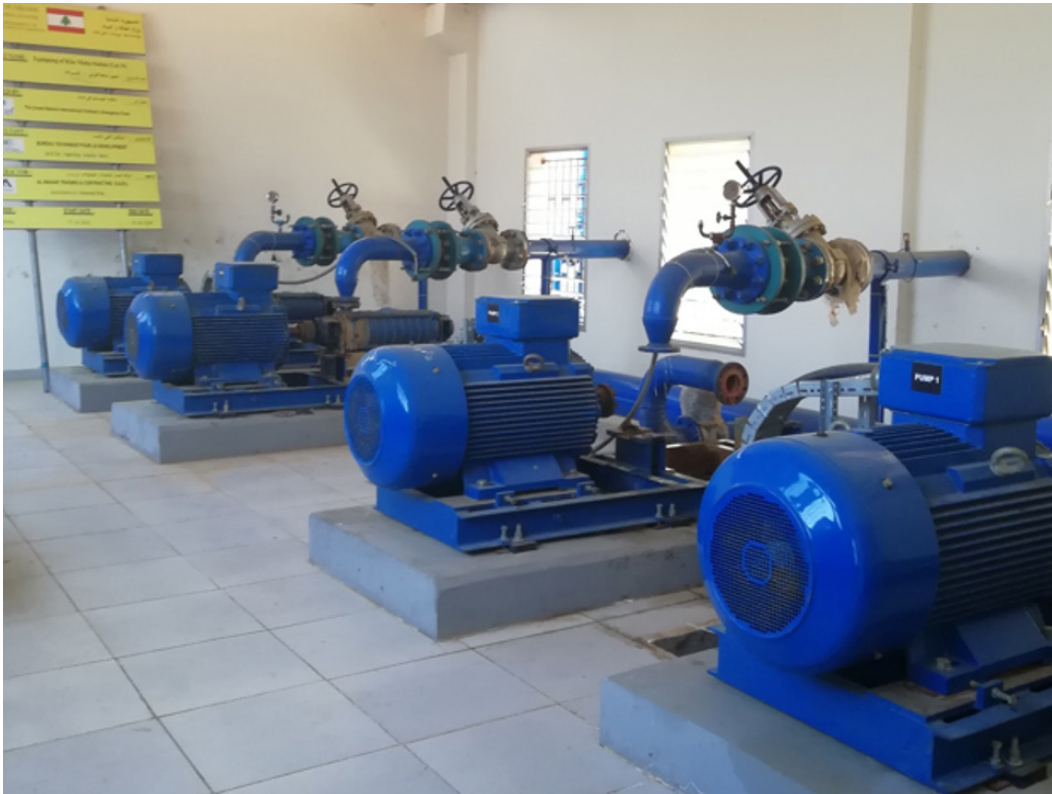
Figure 46. Jisr El Qadi pumping station
