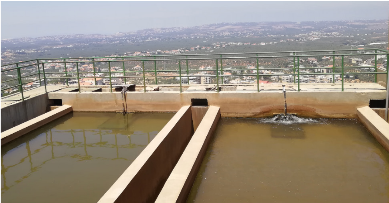
Figure 62. Kousba water treatment plant
