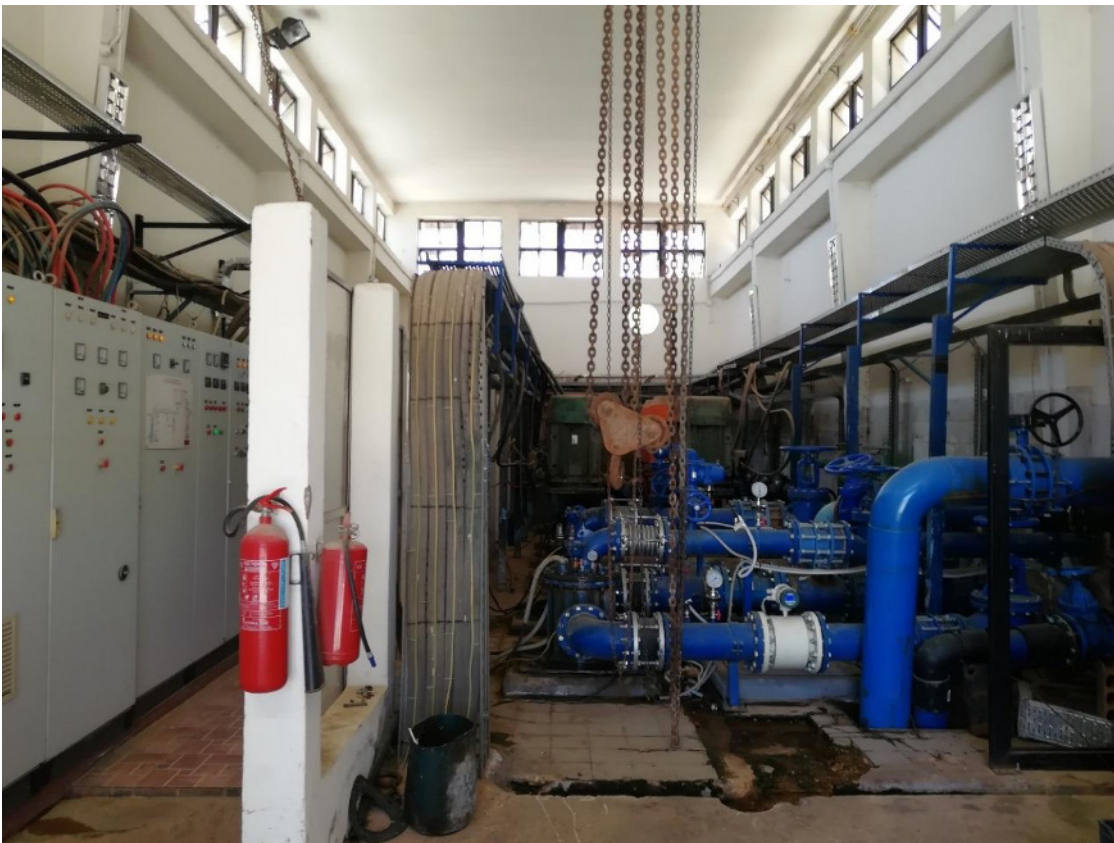
Figure 34. Chamsine water pumping station
